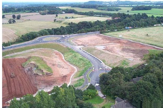
Picture Above: View of new roundabout at A558 Daresbury Expressway, new mini-roundabout on Keckwick Lane and new link road connecting Keckwick Lane with the Daresbury Expressway.
