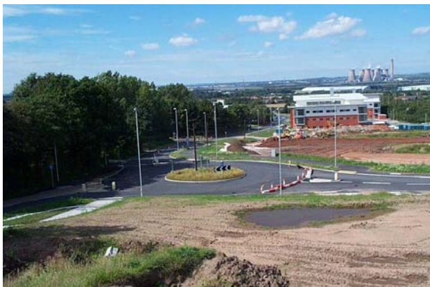
Picture left: View of new roundabout joining Keckwick Lane to A558 Daresbury Expressway
